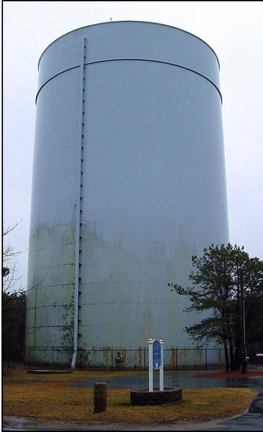
Six-Million Gallon Storage Tank Route 134, South Dennis
