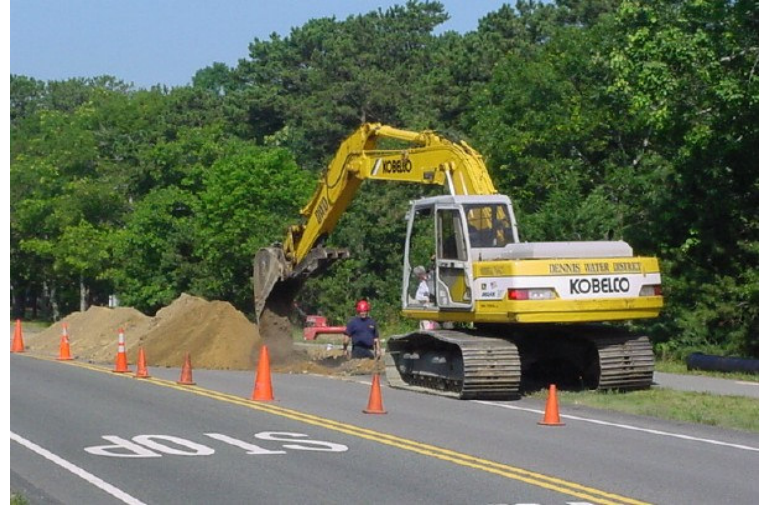
A Dennis Water District work crew installs 12" water main on Setucket Road in July. The District is self-performing all of the raw and treated water main work necessary to connect the 10 wells highest in iron and manganese with the new facilities
